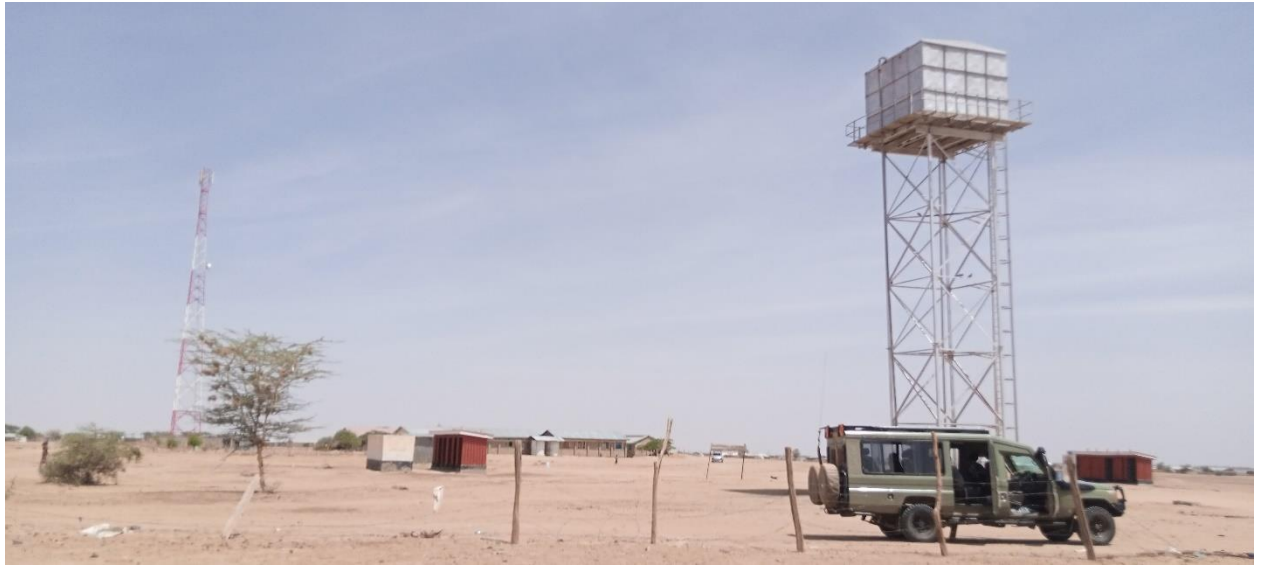
Figure 4-6: Basa Water Project
